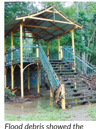
Flood debris showed the creek water had covered all 14 steps to this rotunda at Quota Park, Nambour. Photo: Janine Hill
