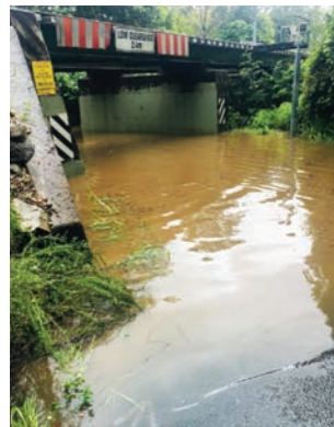
Flooding cut Eudlo School Road, Eudlo. Photo: Michelle Crow
